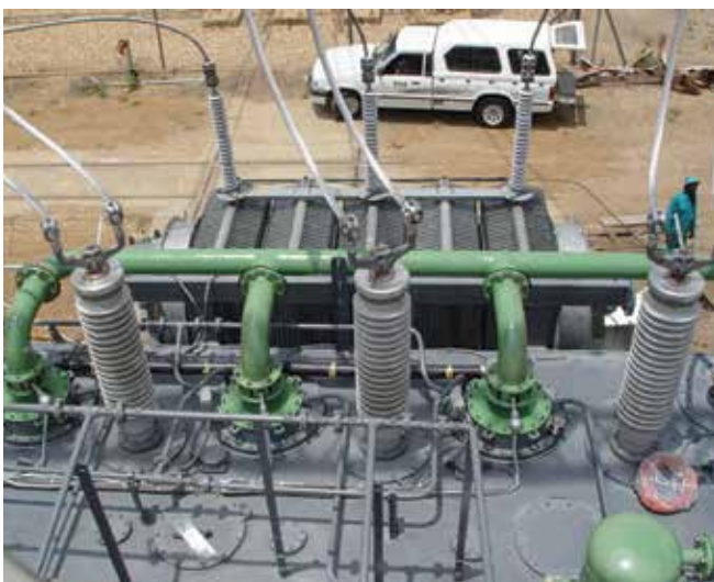
An aerial view of the 220/66-kV, 160-MVA transformer at Van Eck substation shows the protection system discharge of an oil-gas mixture as a result of a dynamic pressure event caused by an internal fault.
