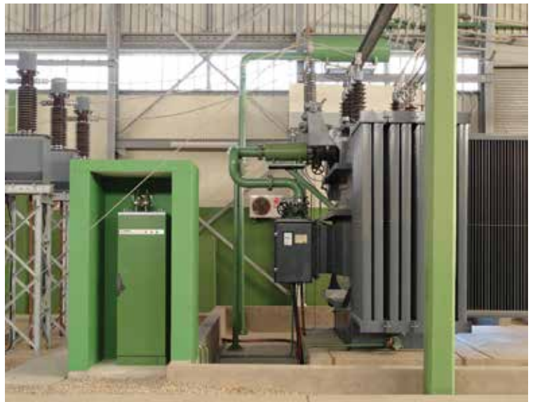
The Sergi transformer protection is installed on the indoor 66/11-kV, 30-MVA transformer at Tamarisk substation, with the nitrogen cabinet located to the left of the transformer.
