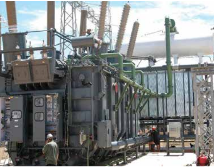
The Zambezi outdoor substation features a 400/220-kV, 315-MVA transformer; the green piping is part of the equipment fire protection system.
