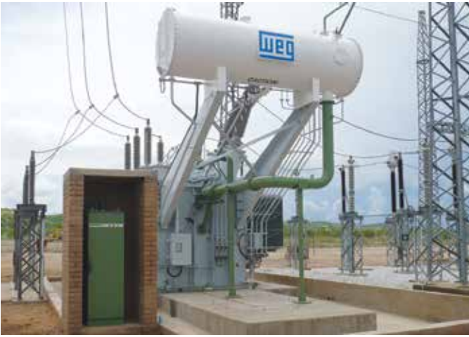
The nitrogen cabinet is evident in this fire protection configuration for the 220/132-kV, 120-MVA transformer at Otjikoto.
