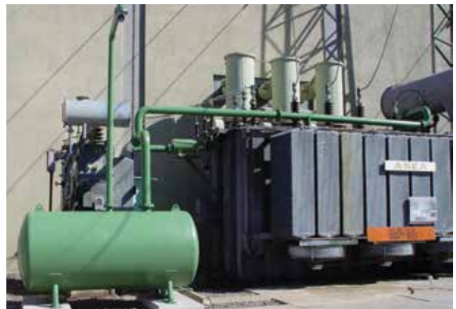
In 2000, NamPower installed three Sergi transformer protection systems on the 330/66-kV, 40-MVA transformers at the Ruacana Hydro Power Plant.
