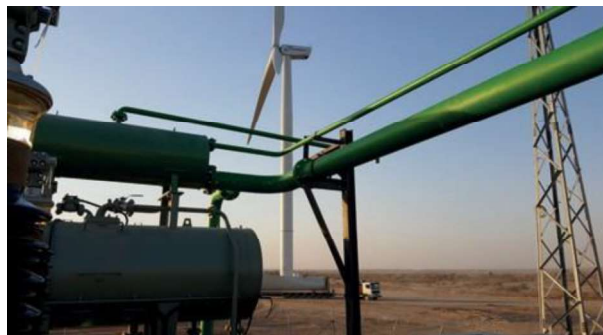
TP system installed on a wind farm
