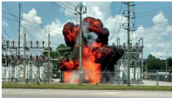
A transformer explosion can have very serious consequences
