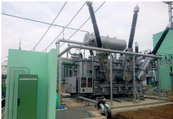
TP system installed on transformer
